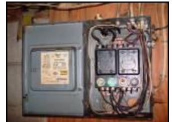
Old 60 Amp Fuse Box
