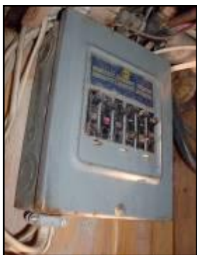
Old Circuit Breaker Box
