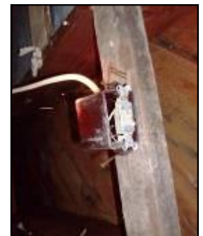
Missing Switch Cover
