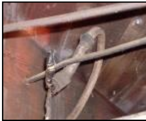
Unsafe Taped Wiring
