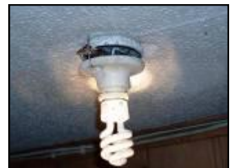
Broken Light Fixture
